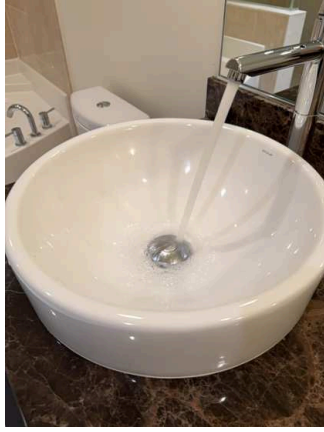
All drains run smoothly (no standing water) (2/2) 02/05/2026 5:21 AM
