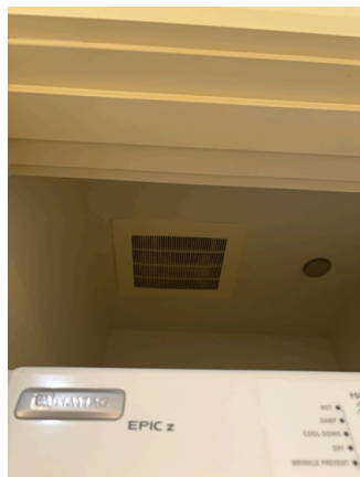
All ventilation fans in laundry room, bathrooms, and kitchen functional (1/2) 02/05/2026 5:20 AM
