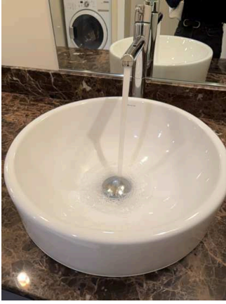
All drains run smoothly (no standing water) (1/2) 02/05/2026 5:21 AM
