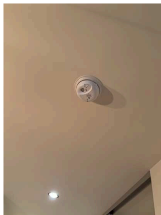
Smoke detectors installed & no beeping (1/2) 02/05/2026 5:13 AM
