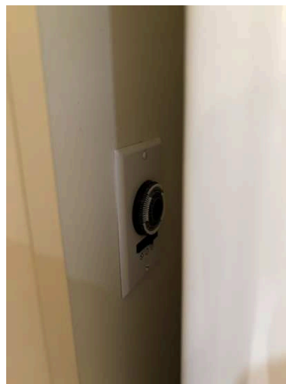
All ventilation fans in laundry room, bathrooms, and kitchen functional (2/2) 02/05/2026 5:20 AM
