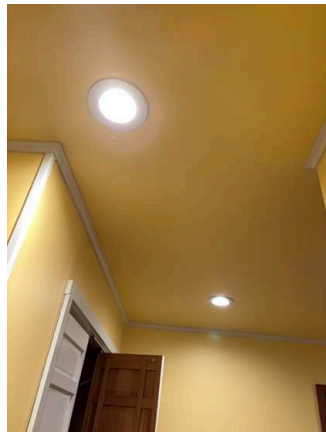
Light fixtures (7/21) 02/02/2026 10:58 AM
