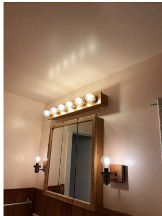
Light fixtures (8/21) 02/02/2026 10:58 AM
