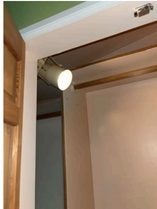
Light fixtures (20/21) 02/02/2026 11:25 AM
