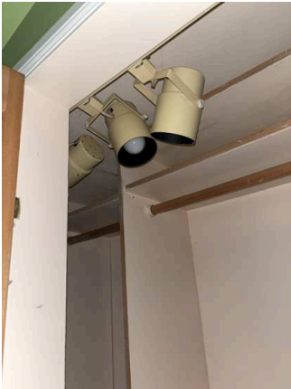
Light fixtures (18/21) 02/02/2026 11:24 AM
