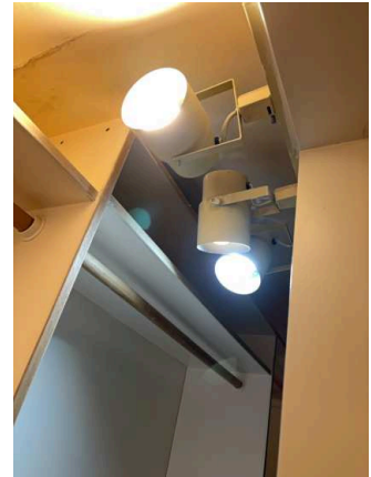
Light fixtures (21/21) 02/02/2026 11:25 AM
