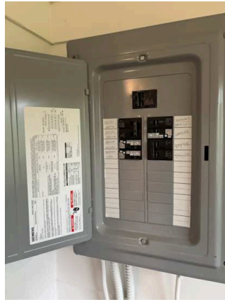
Electrical Panel (1/2) 02/02/2026 10:49 AM
