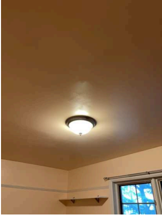
Light fixtures (14/21) 02/02/2026 10:58 AM
