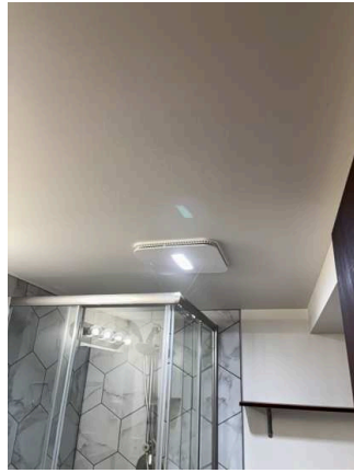
Light fixtures (4/21) 02/02/2026 10:43 AM
