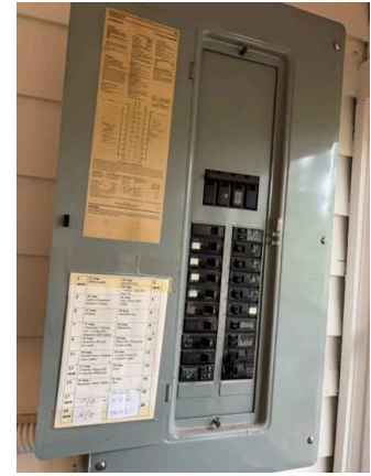
Electrical Panel (2/2) 02/02/2026 10:49 AM
