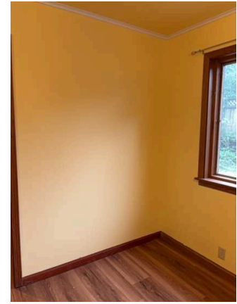
Walls throughout property (20/49) 02/02/2026 11:13 AM
