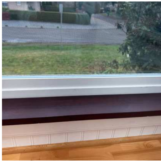
Window sill continued (8/9) 01/15/2026 10:04 AM
