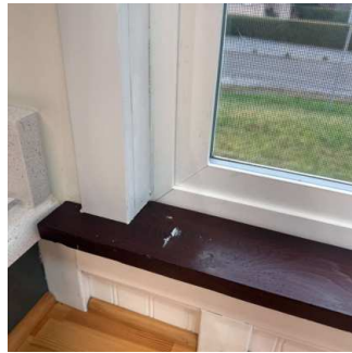
Window sill continued (9/9) 01/15/2026 10:04 AM
