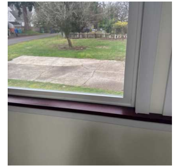
Window Sill (11/16) 01/15/2026 10:02 AM
