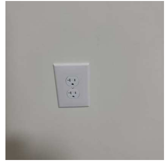
Switches and outlets continued (8/16) 01/15/2026 9:52 AM
