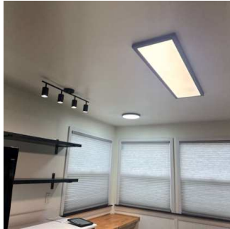
Light fixtures (9/10) 01/15/2026 9:57 AM
