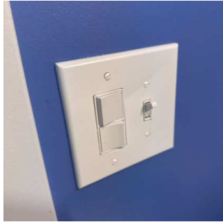
Switches and outlets continued (10/16) 01/15/2026 9:53 AM
