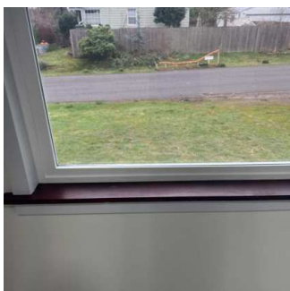
Window Sill (16/16) 01/15/2026 10:03 AM
