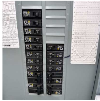
Electrical Panel (3/4) 01/15/2026 10:55 AM
