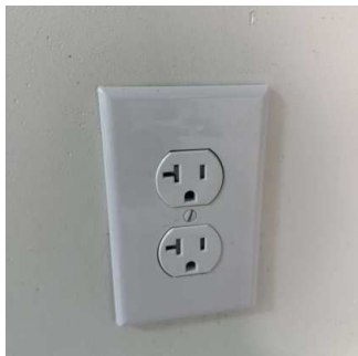
Switches and outlets continued 2 (2/5) 01/15/2026 9:54 AM
