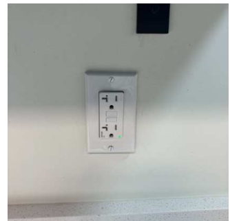
Switches and outlets continued 2 (4/5) 01/15/2026 9:54 AM
