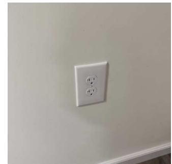
Switches and outlets continued (4/16) 01/15/2026 9:52 AM
