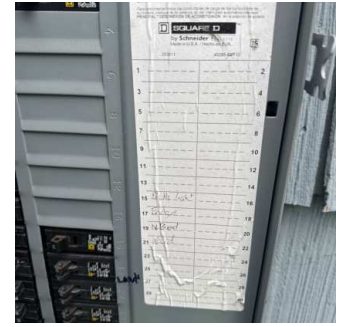
Electrical Panel (4/4) 01/15/2026 10:55 AM
