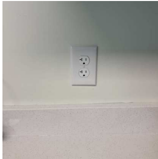
Switches and outlets continued (15/16) 01/15/2026 9:53 AM
