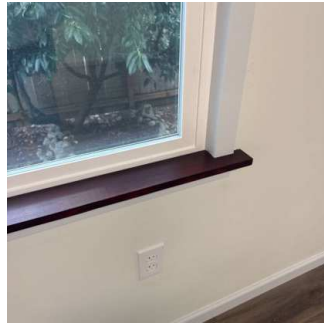
Window Sill (5/16) 01/15/2026 10:02 AM
