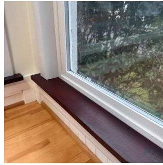
Window sill continued (6/9) 01/15/2026 10:04 AM
