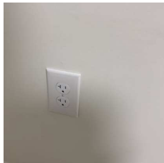
Switches and outlets continued (2/16) 01/15/2026 9:52 AM
