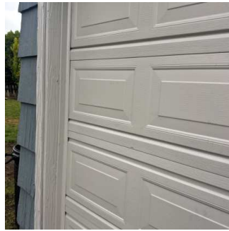
Garage Doors / Openers (2/6) 01/15/2026 10:27 AM
