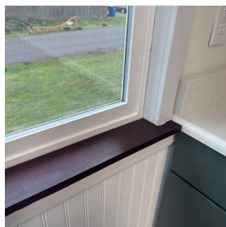
Window sill continued (1/9) 01/15/2026 10:03 AM
