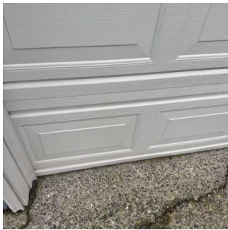
Garage Doors / Openers (5/6) 01/15/2026 10:27 AM
