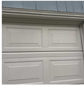
Garage Doors / Openers (3/6) 01/15/2026 10:27 AM
