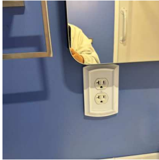
Switches and outlets continued (11/16) 01/15/2026 9:53 AM
