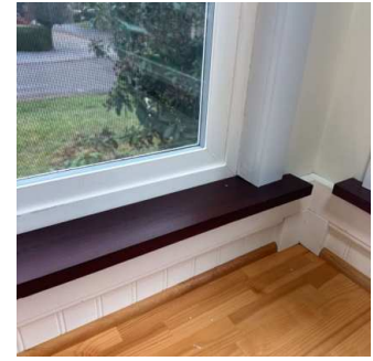
Window sill continued (7/9) 01/15/2026 10:04 AM
