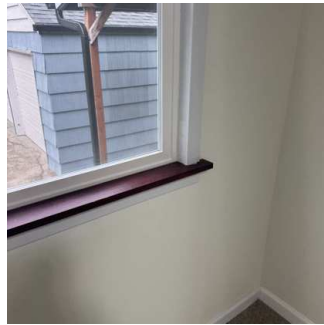
Window Sill (9/16) 01/15/2026 10:02 AM
