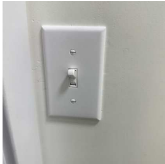
Switches and outlets continued (14/16) 01/15/2026 9:53 AM
