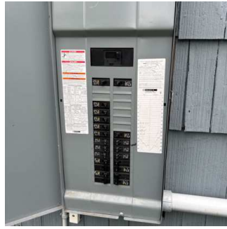
Electrical Panel (2/4) 01/15/2026 10:55 AM
