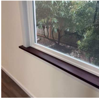
Window Sill (4/16) 01/15/2026 10:02 AM
