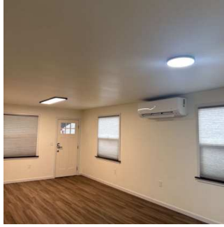
Light fixtures (2/10) 01/15/2026 9:56 AM
