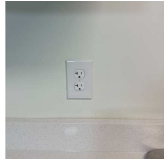
Switches and outlets continued (16/16) 01/15/2026 9:53 AM
