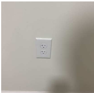
Switches and outlets continued (1/16) 01/15/2026 9:52 AM
