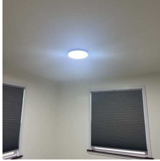
Light fixtures (6/10) 01/15/2026 9:56 AM
