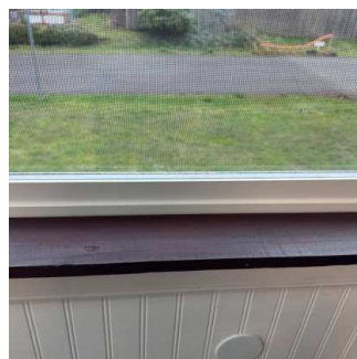
Window sill continued (2/9) 01/15/2026 10:03 AM
