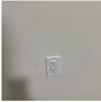
Switches and outlets continued (6/16) 01/15/2026 9:52 AM
