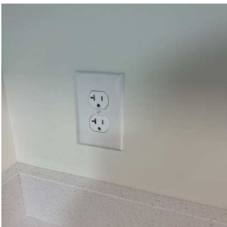
Switches and outlets continued 2 (1/5) 01/15/2026 9:54 AM
