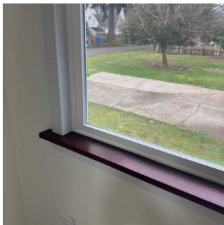
Window Sill (12/16) 01/15/2026 10:02 AM
