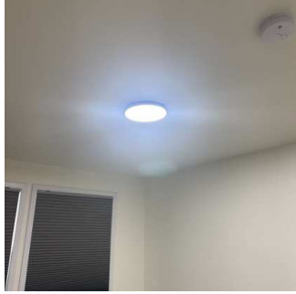
Light fixtures (5/10) 01/15/2026 9:56 AM
