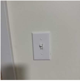
Switches and outlets continued (5/16) 01/15/2026 9:52 AM
