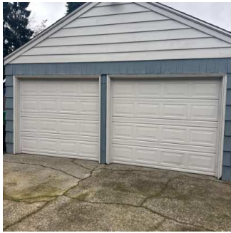
Garage Doors / Openers (1/6) 01/15/2026 10:27 AM
