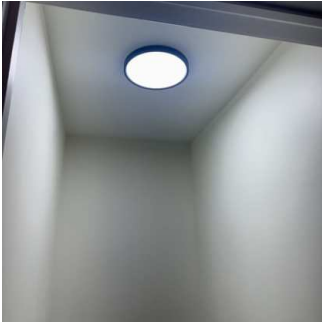
Light fixtures (8/10) 01/15/2026 9:56 AM
