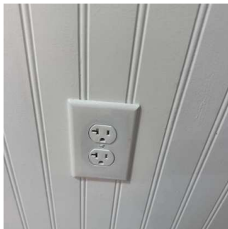
Switches and outlets continued 2 (3/5) 01/15/2026 9:54 AM
