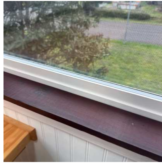
Window sill continued (5/9) 01/15/2026 10:03 AM
