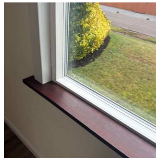
Window Sill (2/16) 01/15/2026 10:02 AM
