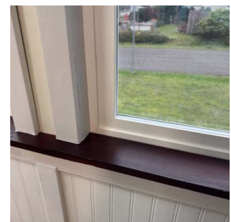
Window sill continued (3/9) 01/15/2026 10:03 AM
