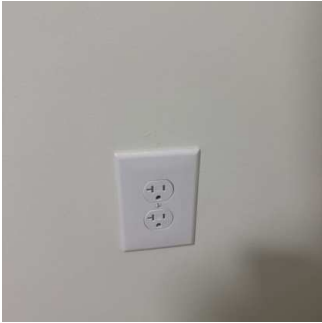
Switches and outlets continued (9/16) 01/15/2026 9:52 AM
