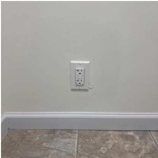
Switches and outlets continued (13/16) 01/15/2026 9:53 AM
