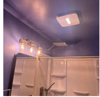
Light fixtures (7/10) 01/15/2026 9:56 AM
