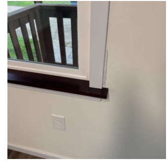
Window Sill (7/16) 01/15/2026 10:02 AM
