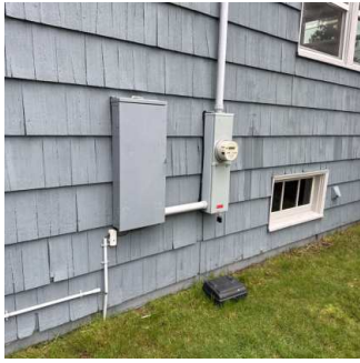
Electrical Panel (1/4) 01/15/2026 10:55 AM
