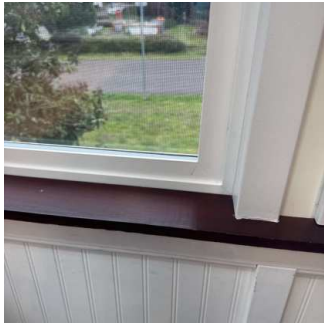
Window sill continued (4/9) 01/15/2026 10:03 AM
