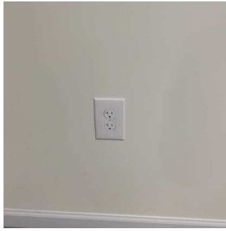
Switches and outlets continued (7/16) 01/15/2026 9:52 AM
