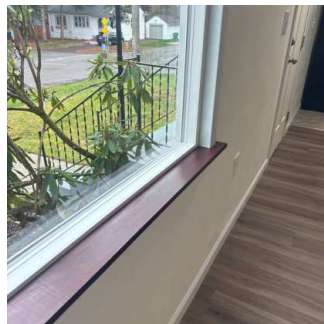
Window Sill (1/16) 01/15/2026 10:02 AM
