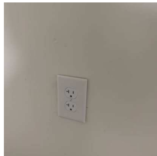
Switches and outlets continued (3/16) 01/15/2026 9:52 AM
