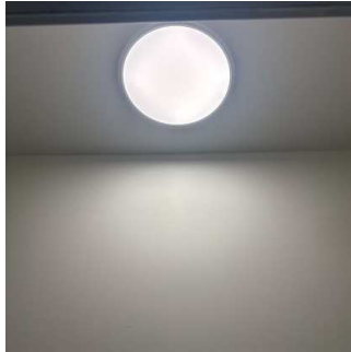
Light fixtures (10/10) 01/15/2026 9:57 AM
