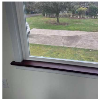
Window Sill (14/16) 01/15/2026 10:03 AM
