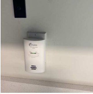
Switches and outlets continued 2 (5/5) 01/15/2026 9:54 AM
