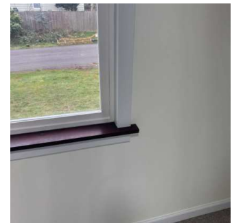
Window Sill (15/16) 01/15/2026 10:03 AM
