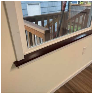
Window Sill (8/16) 01/15/2026 10:02 AM
