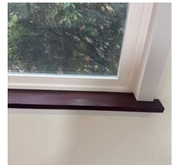
Window Sill (3/16) 01/15/2026 10:02 AM
