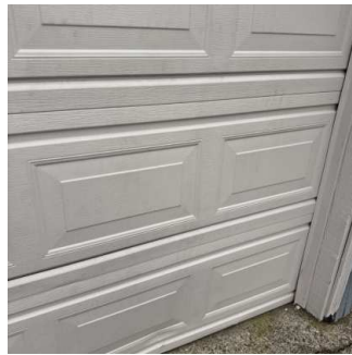
Garage Doors / Openers (6/6) 01/15/2026 10:27 AM
