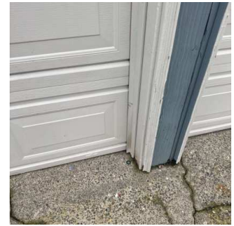
Garage Doors / Openers (4/6) 01/15/2026 10:27 AM
