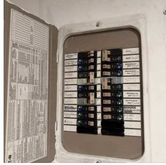
Electrical Panel (Photo Required) (1/2) 09/18/2025 1:12 PM
