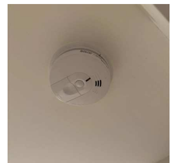
Test all smoke alarms in all bedrooms + kitchen? (Photo Required) (3/3) 09/18/2025 1:11 PM
