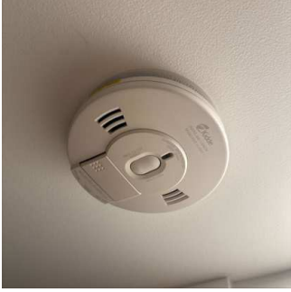
Test CO detectors on all levels (Photo Required) 09/18/2025 1:11 PM
