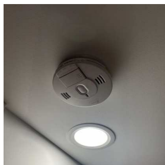
Test all smoke alarms in all bedrooms + kitchen? (Photo Required) (1/3) 09/18/2025 1:10 PM
