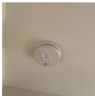
Test all smoke alarms in all bedrooms + kitchen? (Photo Required) (2/3) 09/18/2025 1:11 PM
