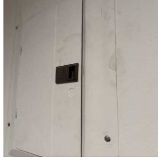
Electrical Panel (Photo Required) (2/2) 09/18/2025 1:13 PM
